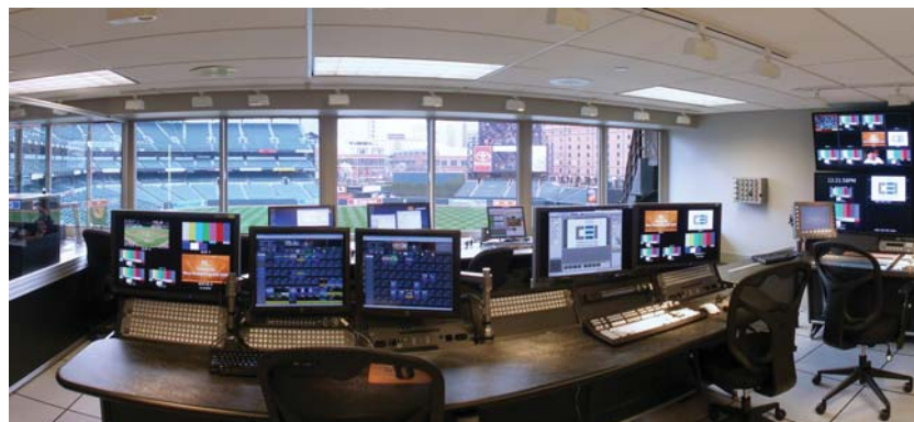
The scoreboard control room at Oriole Park at Camden Yards.
